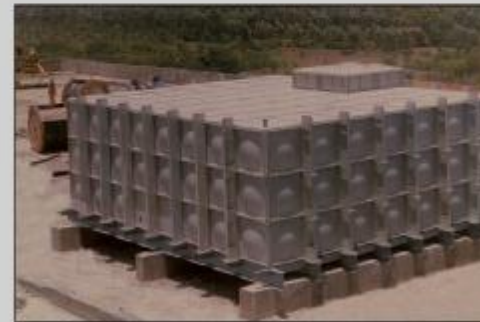
3m. Deep 168 KL tank for Drinking water at the terrace of an InfoTech Building
