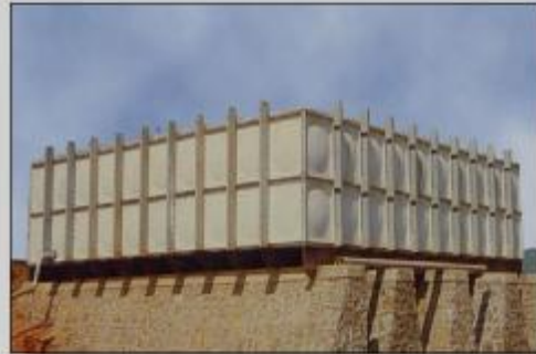
2m. Deep 200 KL tank for Raw water at a Irrigation site
