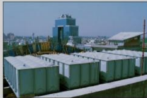
70 KL, 56 KL 2x42 KL for raw and drinking water at a Shopping Complex
